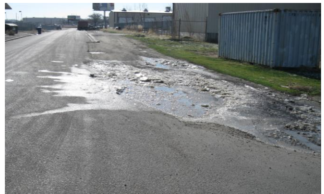
Damaged Street Edges
