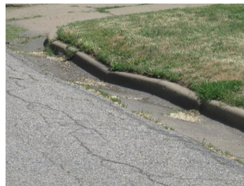
Damaged Curb and Gutter
